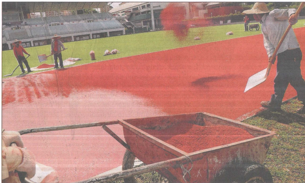
Workers re-surfacing the running track at the Bishan Stadium, which will also get a new lighting system. ST PHOTO: JOYCE FANG
